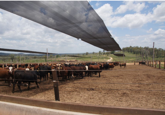
Shade sails should be pulled taut and twisted so one axis is convex and the other axis concave. Shapes with little curvature and tension will deform under load and become unstable. Sloping fabric will ensure good shedding of water and hail.
