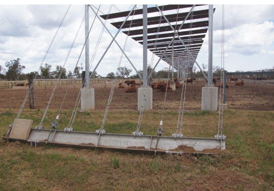
Shading material is often supported on cable suspended between columns, posts or supports. Infrastructure must be engineered for rain, hail and wind loadings.
