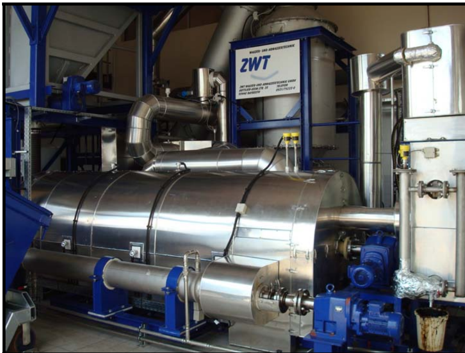
Figure 4.7: ZWT Pyrolyser at Mintraching, Germany
