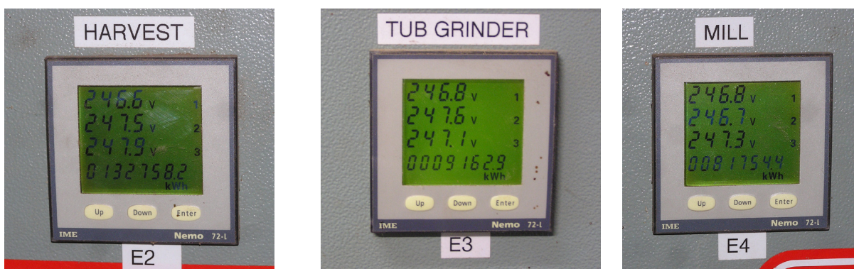
Photograph 27 - Installed power meters E2, E3 and E4 at Feedlot B
