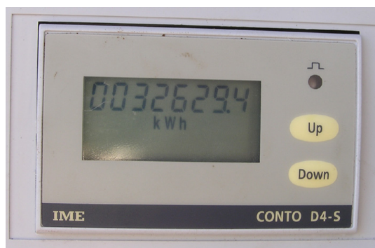
Photograph 24 - IME CONTO D4-S power meter
