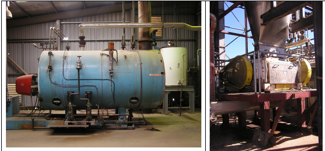
Photograph 2 - Typical steam flaking system - Boiler (Left) and Steam Chest (Right)
