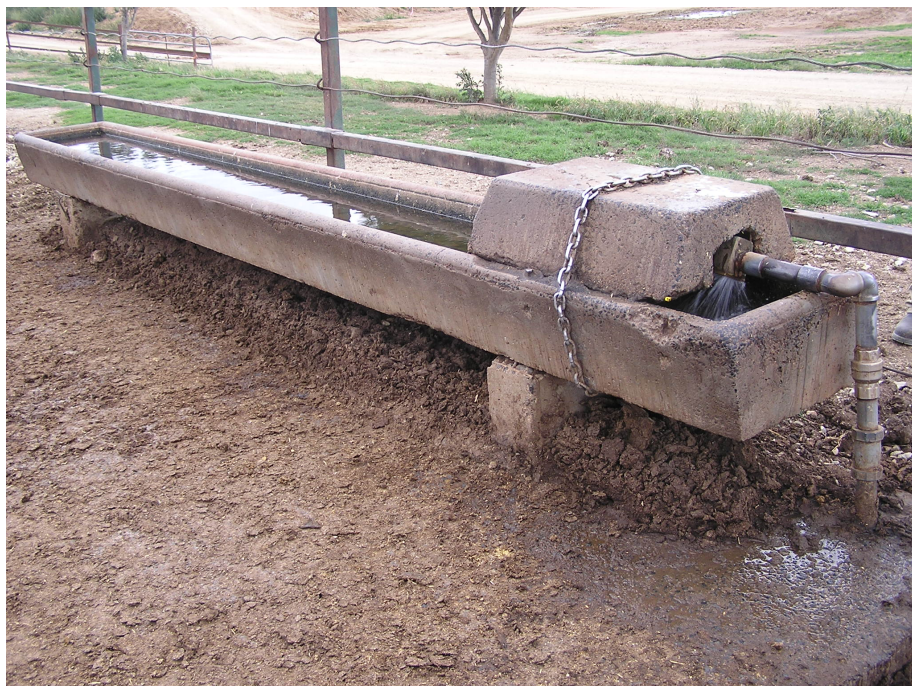
Photograph 59 – Old Type-1 style trough with trapezoidal cross-section and concrete float valve cover (Feedlot F)
