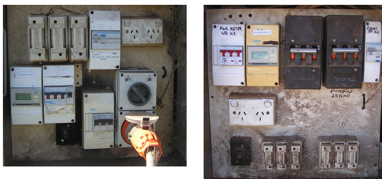
Photograph 32 - Installed power meters E13 and E14 at Feedlot D
