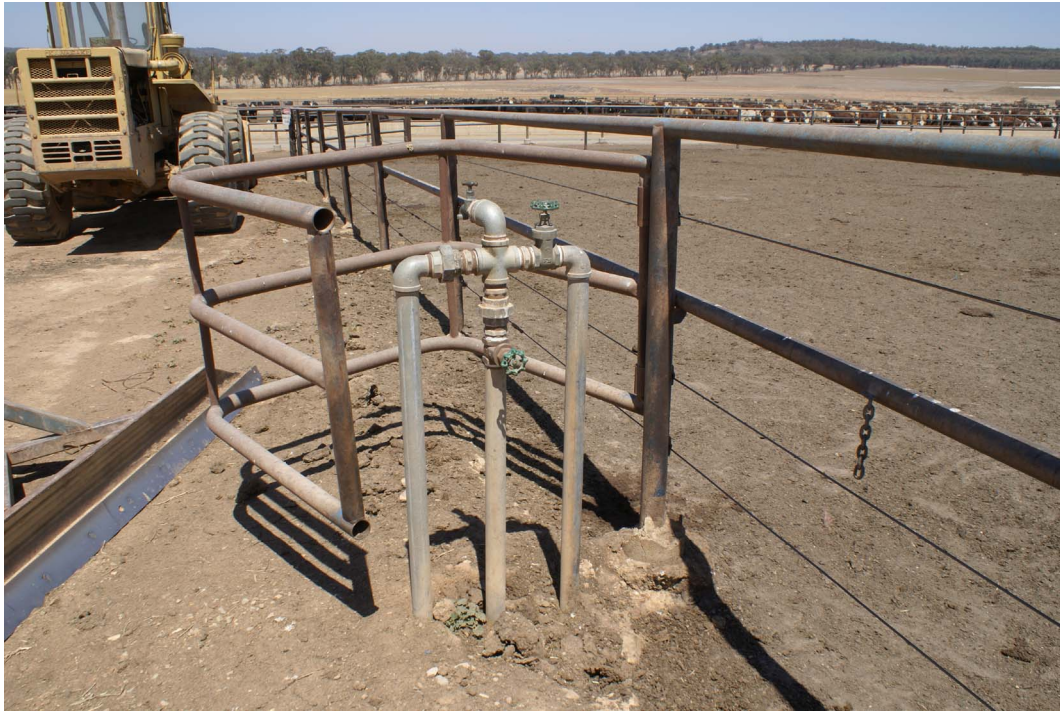
Photograph 52 – Pipe & valves used to flush sewer line (Feedlot B)
