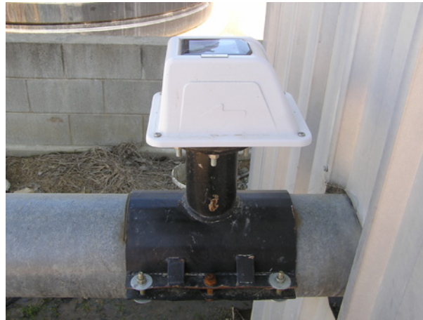
Photograph 38 – Installed water meter M2 and data logger at Feedlot F
