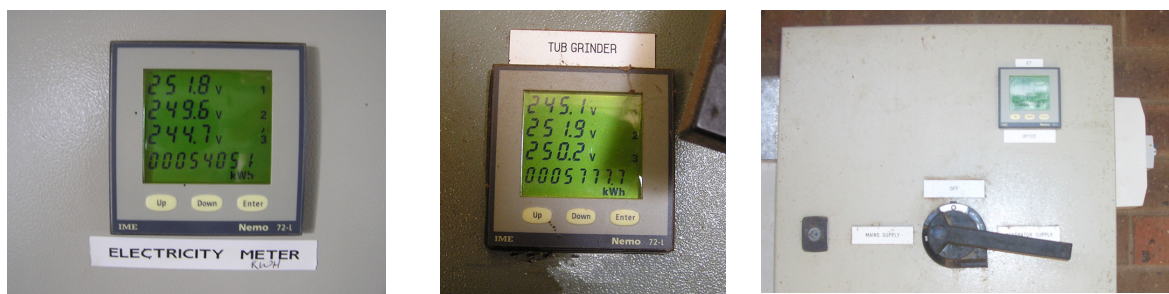
Photograph 37 - Installed power meters E4, E5 and E8 at Feedlot H
