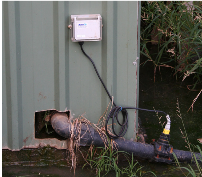
Photograph 25 – Installed water meter M6 at Feedlot A
