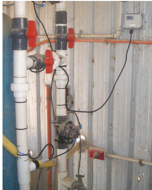
Photograph 40 – Installed water meter M4 at Feedlot F
