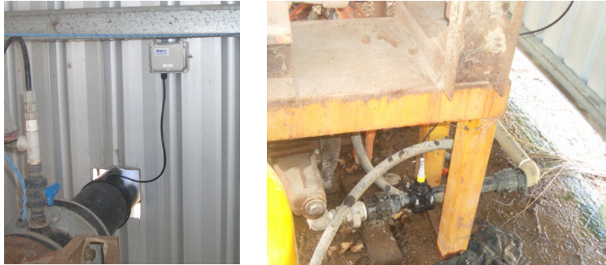
Photograph 39 – Installed water meter M3 at Feedlot F
