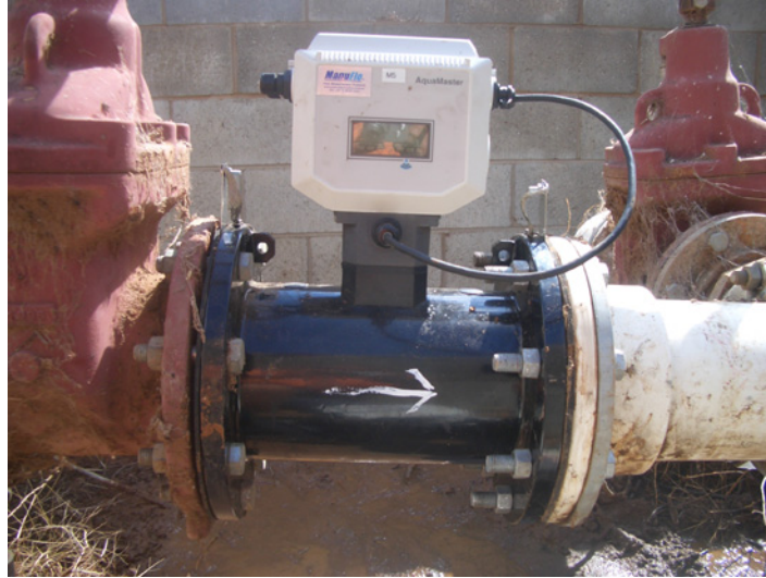
Photograph 31 – Installed water meter M5 at Feedlot C
