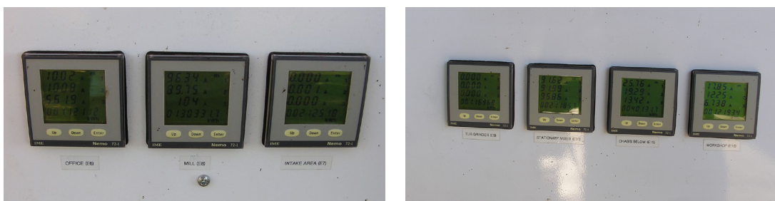
Photograph 30 - Installed power meters E6, E7, E8 (Left) and E9, E10, E15, E16 (Right) at Feedlot D
