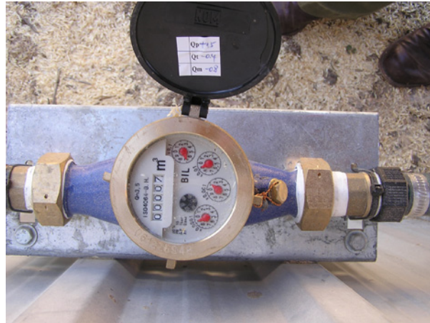
Photograph 46 – Installed water meter M2 at Feedlot H
