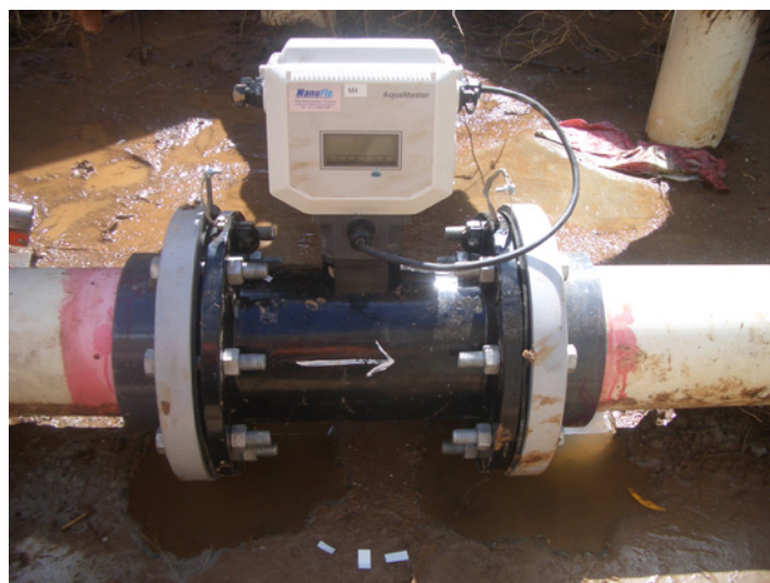
Photograph 30 – Installed water meter M4 at Feedlot C
