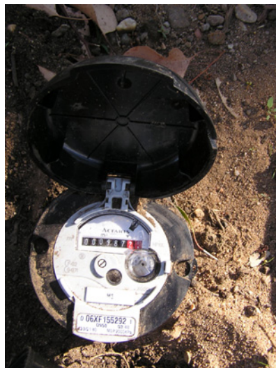
Photograph 45 – Installed water meter M1 at Feedlot H
