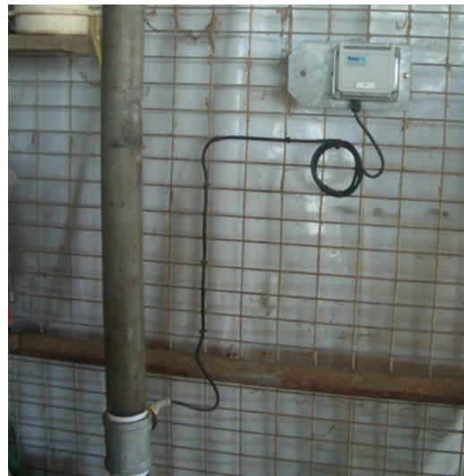
Photograph 41 – Installed water meter M5 at Feedlot F
