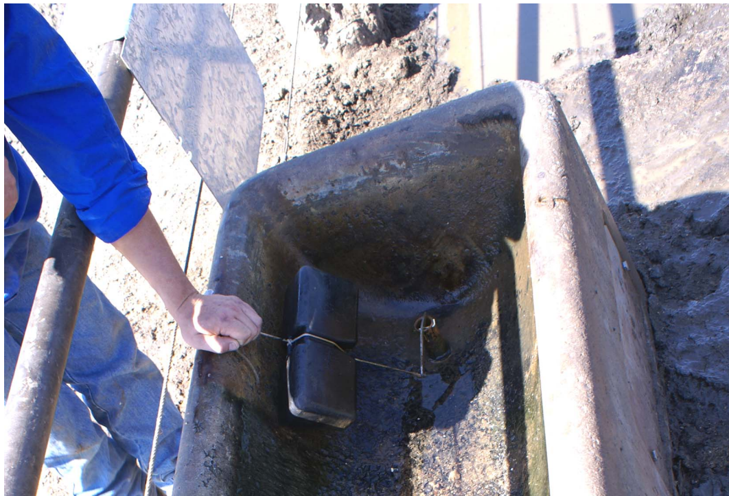
Photograph 51 – Float valve – plastic float on a rope – valve sprays upwards (Feedlot B)
