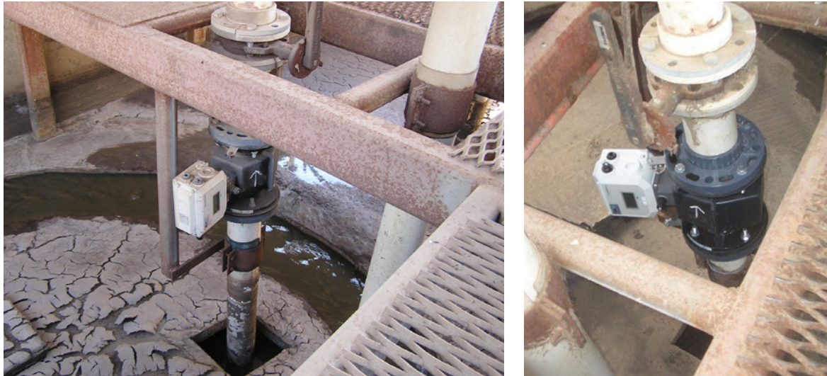
Photograph 34 – Installed water meter M8 at Feedlot C
