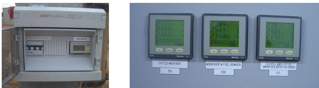
Photograph 36 - Installed power meters E7, E8, E9 and E10 at Feedlot G
