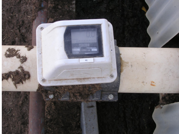
Photograph 42 – Installed water meter M6 at Feedlot F
