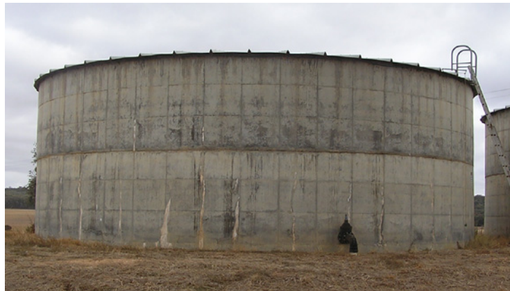
PHOTOGRAPH 15 – ENCLOSED CONCRETE WATER STORAGE TANK
