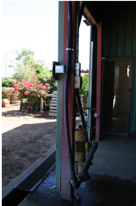
Photograph 26 – Installed water meter M7 at Feedlot A
