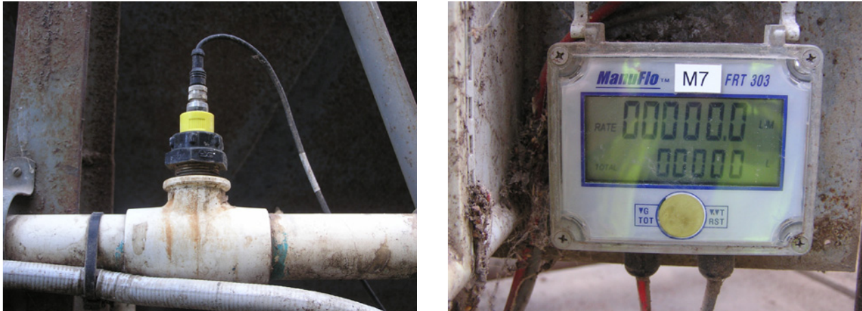
Photograph 37 – Installed water meter M7 at Feedlot E
