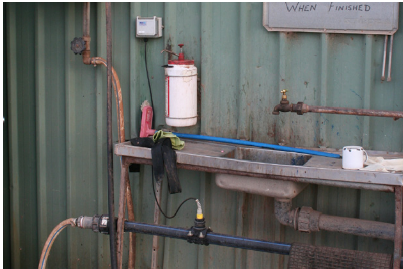
Photograph 23 – Installed water meter M3 at Feedlot A
