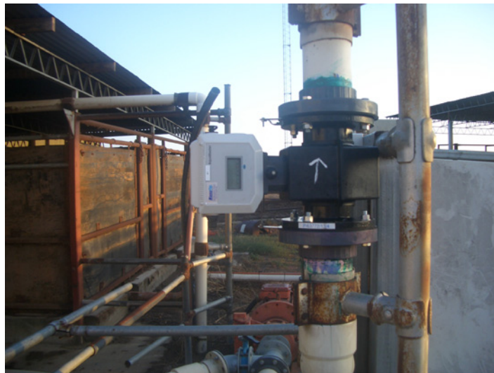
Photograph 33 – Installed water meter M7 at Feedlot C
