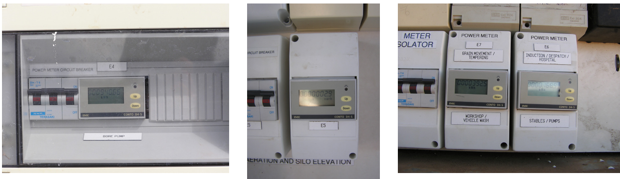
Photograph 33 - Installed power meters E4, E5, E6 and E7 at Feedlot E
