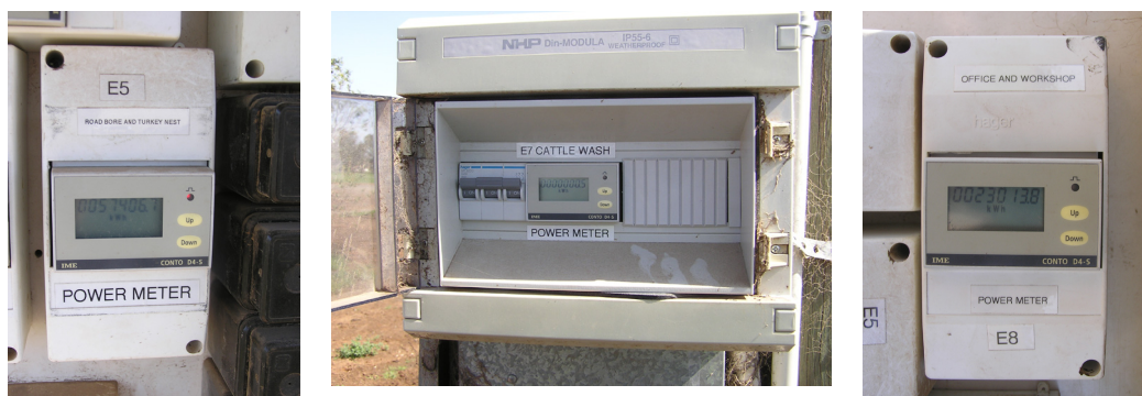
Photograph 28 - Installed power meters E5, E7 and E8 at Feedlot B
