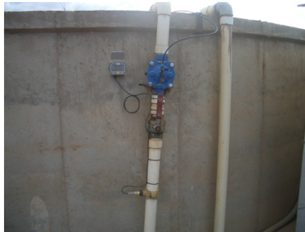
Photograph 28 – Installed water meter M7 at Feedlot B
