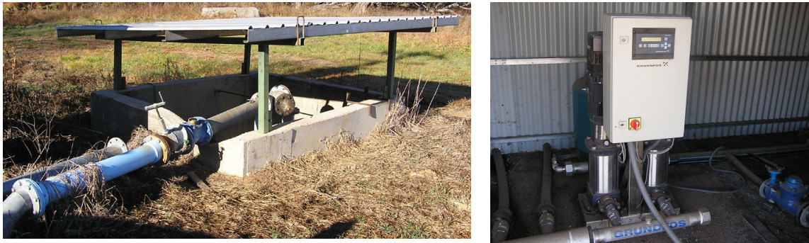
Photograph 15 - Water supply pump (Left) and Reticulation pump station (Right)
