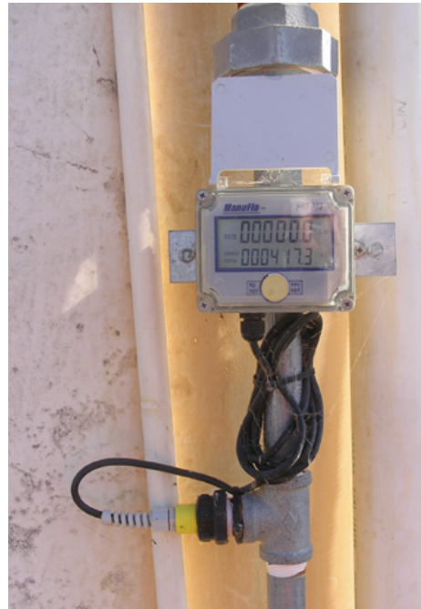
Photograph 43 – Installed water meter M12 at Feedlot F
