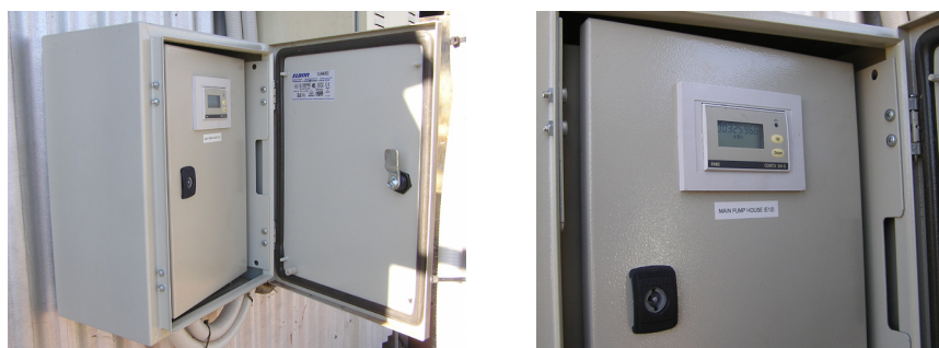
Photograph 31 - Installed power meters E11 and E12 at Feedlot D
