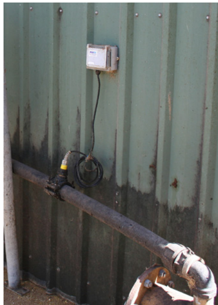
Photograph 24 – Installed water meter M5 at Feedlot A
