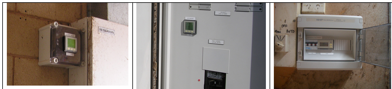
Photograph 38 - Installed power meters E6, E7 and E10 at Feedlot H
