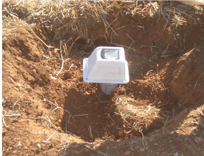
PHOTOGRAPH 32 – INSTALLED WATER METER M6 AT FEEDLOT C
