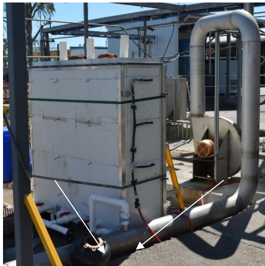
Fig 16: Non-condensables exhaust ducting and offtakes
