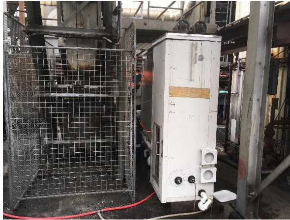
Fig 19: After the scrubber installed
