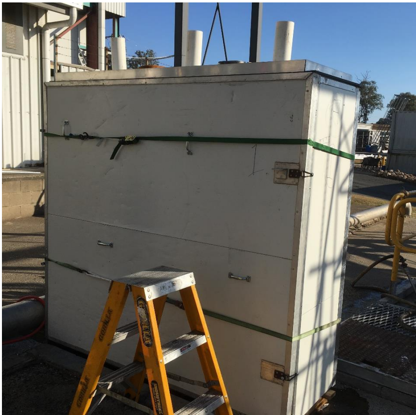
Fig 18: View of pilot Scale biofilter showing door and gas exhaust pipes
