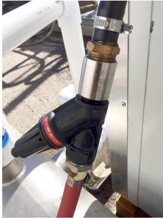
Fig 21: Low flow pressure reduction valve
