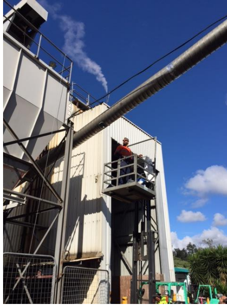
Fig 8: Blood ring-dryer exhaust duct: access can sometimes be an issue.
