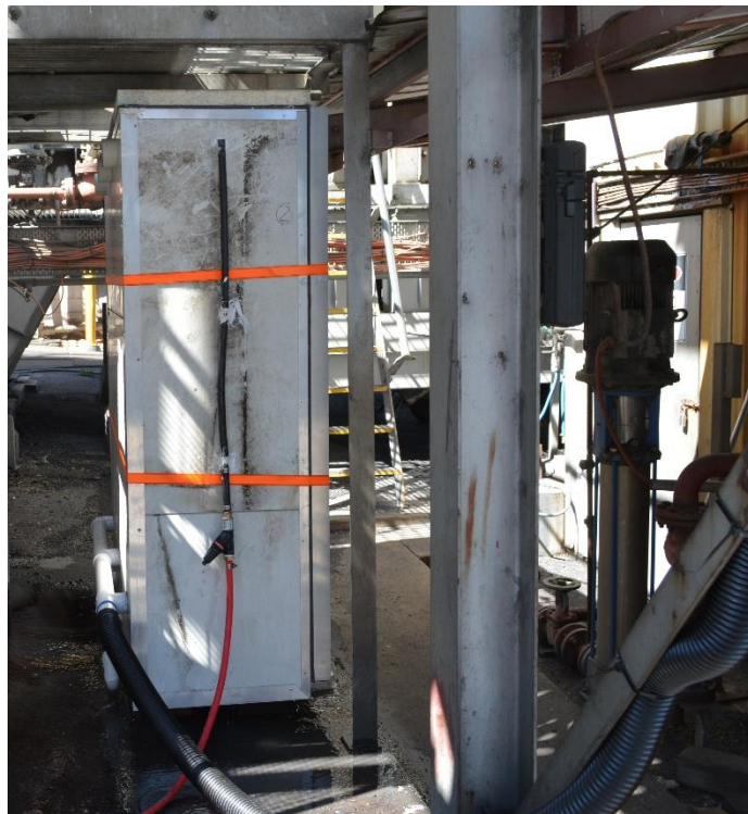
Fig 18: Before the scrubber installed
