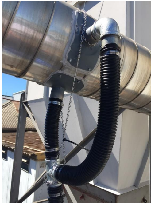
Fig 17: Connection showing flexible hosing
