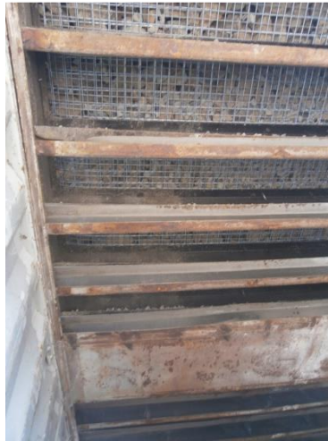
Fig 2: Looking at the underneath of the floor of the top container showing rock fill and supports
