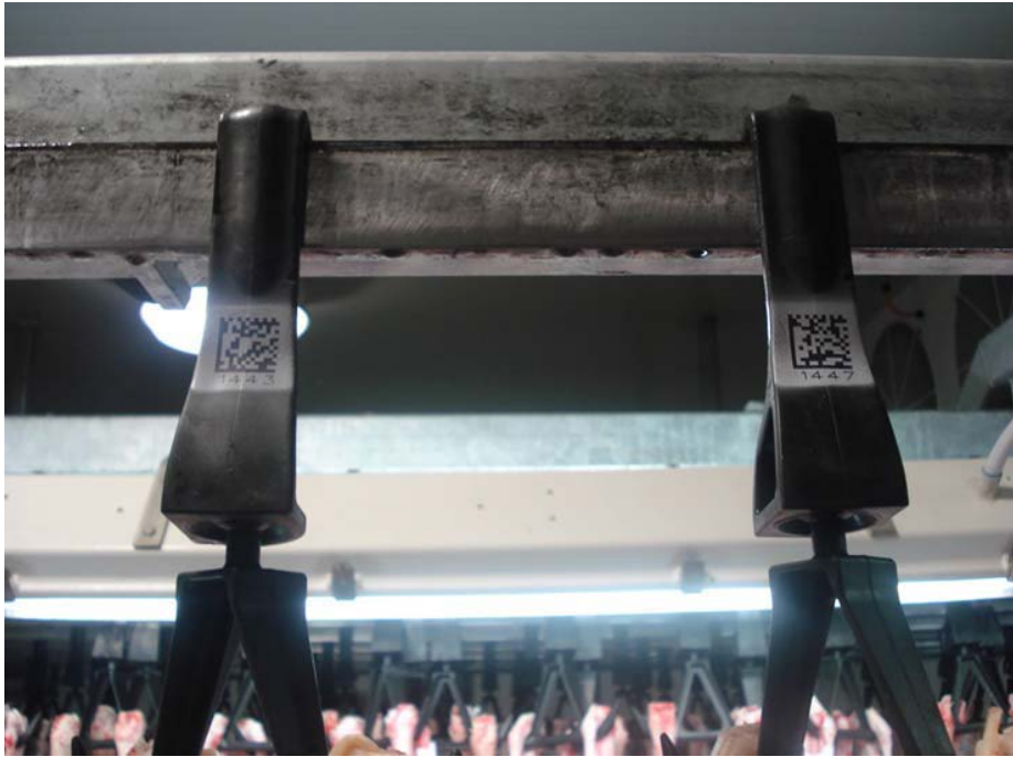
Image 23: Skids in the Chillers
