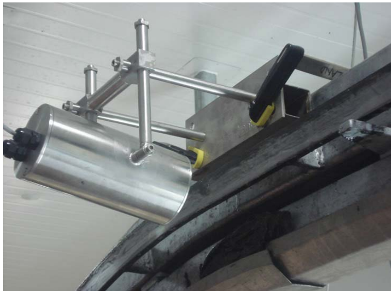
Image 16: Marshalling Area camera mounted on the out-feed conveyor
