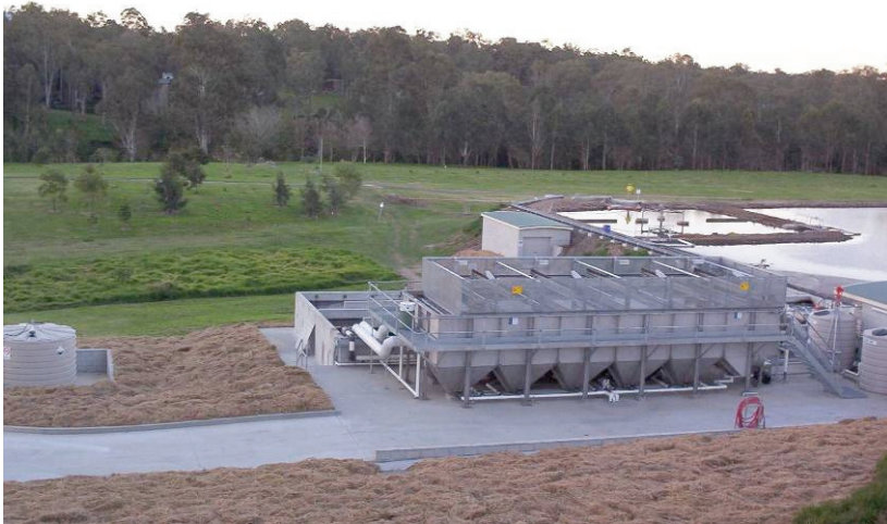
Dinmore's new Tertiary DAF and Disinfection System
