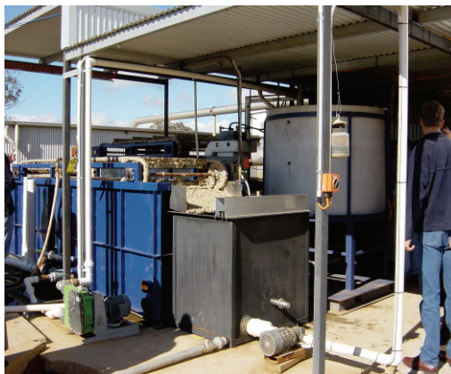
The EC based wastewater treatment plant at Burrangong Abattoirs
