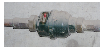
Figure 8: Inline gas flow meter
