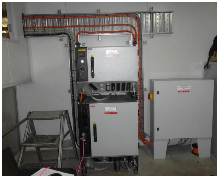
Fig.12 Robots controllers, MCC and cabling in control room
