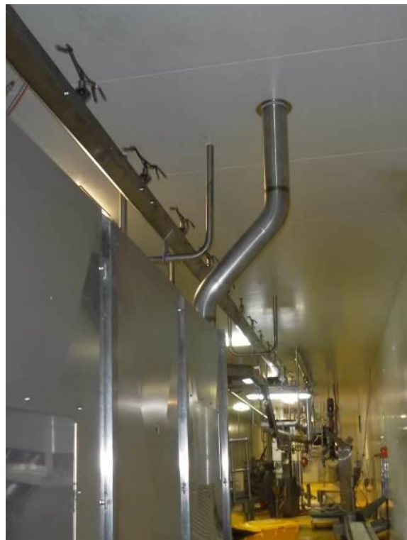
Fig.10 Dog leg required in robot conduit to avoid overhead conveyor
