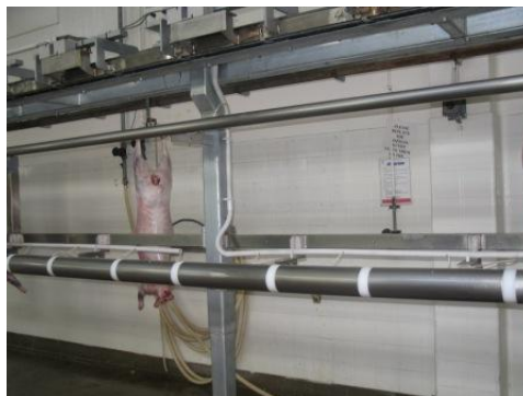
Photo 2. Rail segmented into electrically isolated 8 sections (stimulation sections and 4 test pulse sections) using insulating blocks. Recent installations have shown that these blocks should be no wider than 20mm to avoid issues with carcass bouncing.
