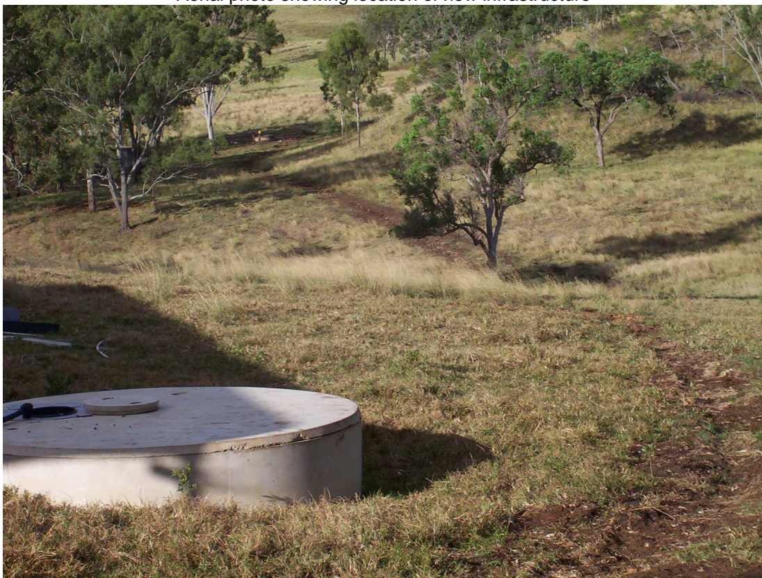
Installation of water pipe using a backhoe. Existing trough in the distance.
