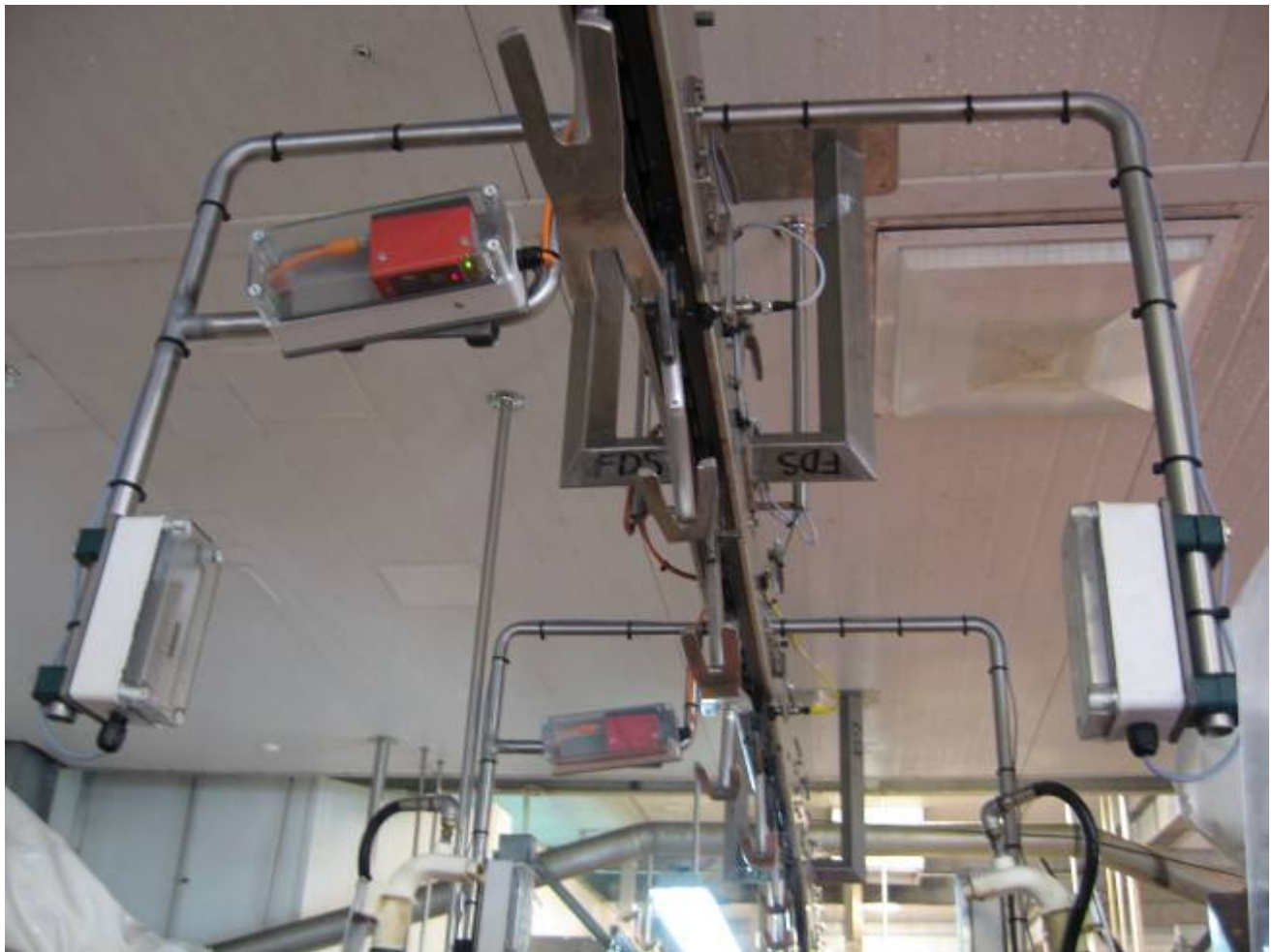
Fig. 6 Sensors mounted at GMP
