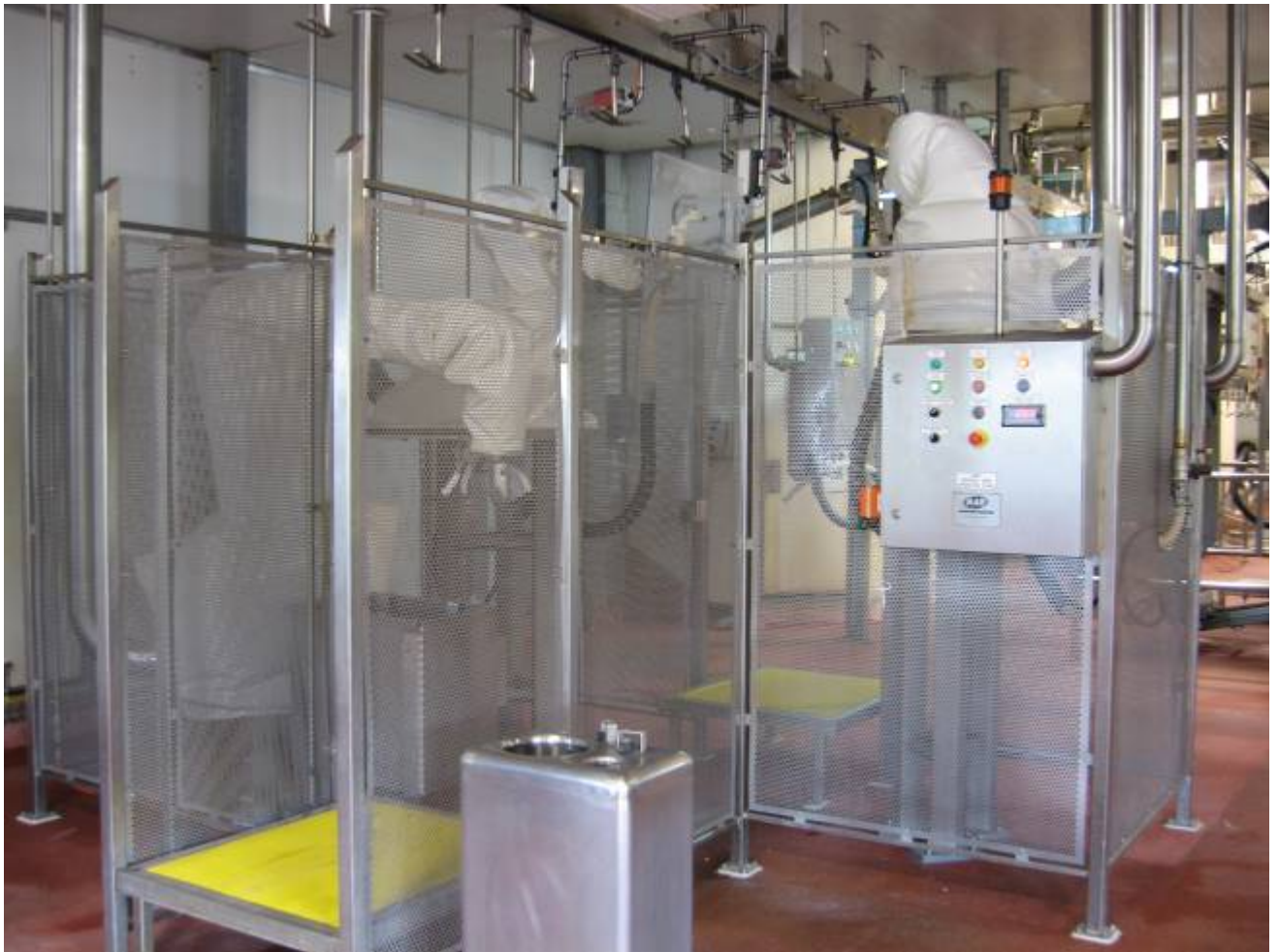
Fig. 4 Cell Perforated guarding installed at GMP
