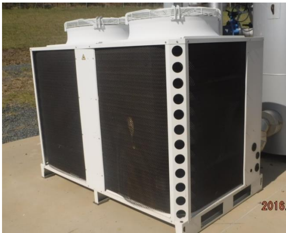
Figure 30. Chiller refrigeration unit
