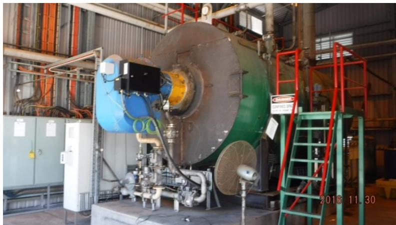
Figure 15. Biogas Boiler (General Electric 4MW)
