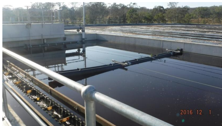
Figure 21. Biolac clarifier for activated sludge settling
