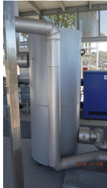
Figure 12. Glycol storage tank
