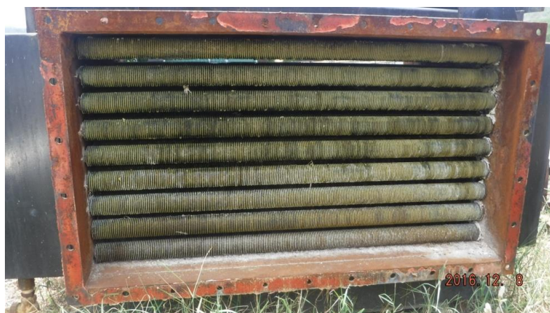
Figure 40. Teys Rockhampton biogas boiler economiser
