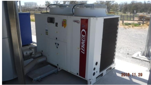
Figure 14. Chiller refrigeration unit
