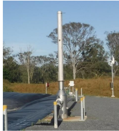
Figure 17. CAL Emergency Vent
