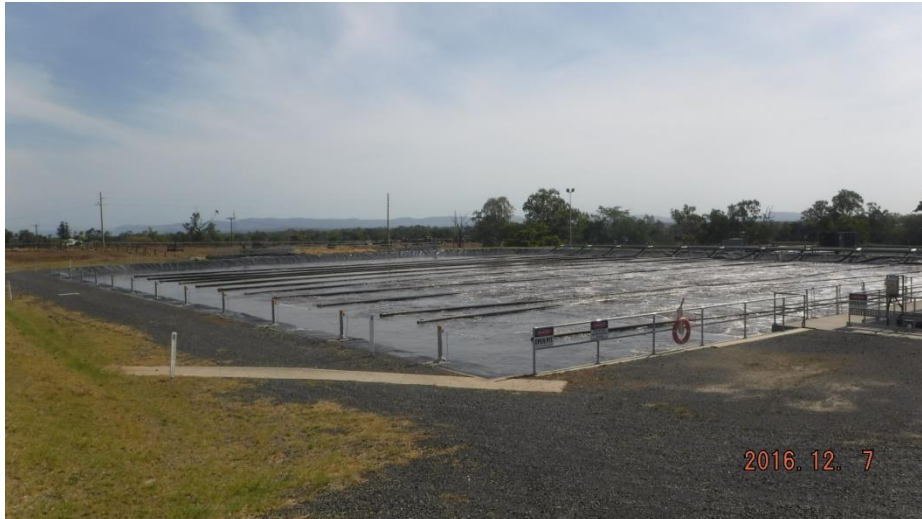
Figure 33. Biolac biological nutrient removal plant
