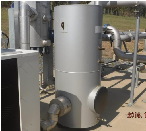
Figure 28. Glycol storage tank
