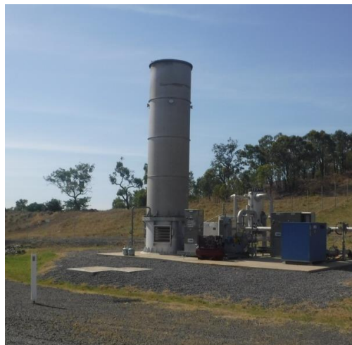
Figure 32. Fully enclosed flare
