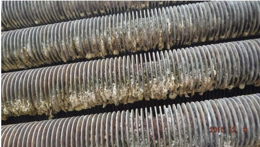
Figure 41. Sulphur deposits on the Teys Rockhampton economiser
