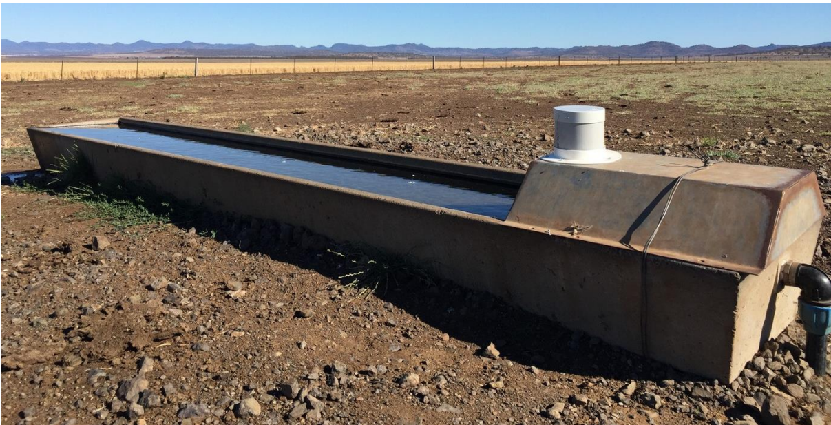
Figure 5: Waterwatch T35 mounted under protective cover
