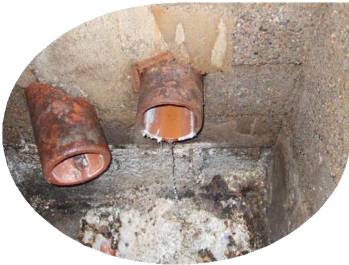
Photo 3. The Boning Room drain. Although only a trickle at the time of the shot, the excellent quality of this flow is clearly seen and is supported by analytical data.
