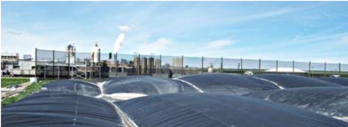
Figure 7 Covered anaerobic lagoon operating under a positive pressure gas collection system
