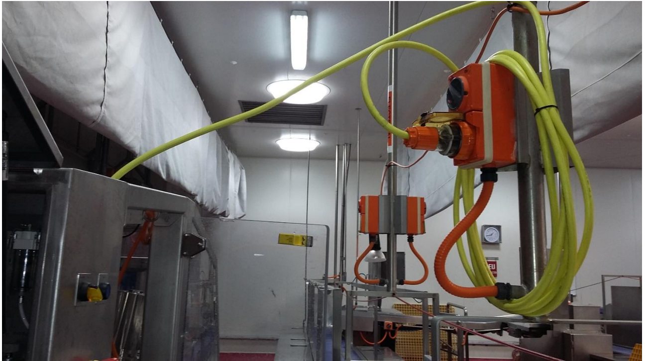
Figure 23: Power supply now enters machine near the top
