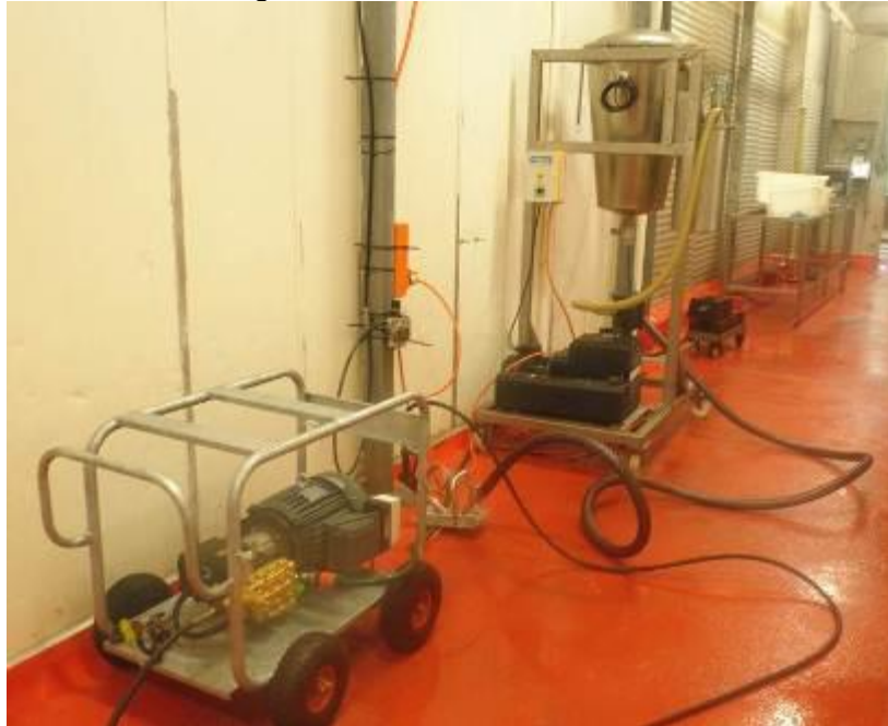
Fig.15 Equipment setup for HP water tool, the HP water unit and vacuum system are shown.
