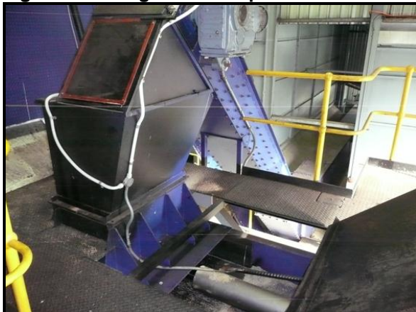
Inclined feed conveyor and ram feeder
