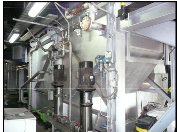
Boiler showing sloping grate
