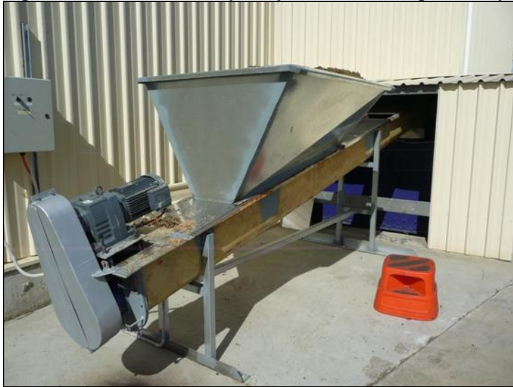
Figure 4.4: Picture of temporary PW+DAF sludge feed system
