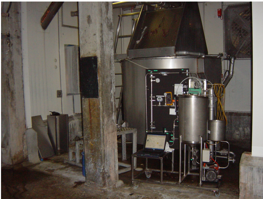
Figure 8: Catchment tank at Casino abattoir
