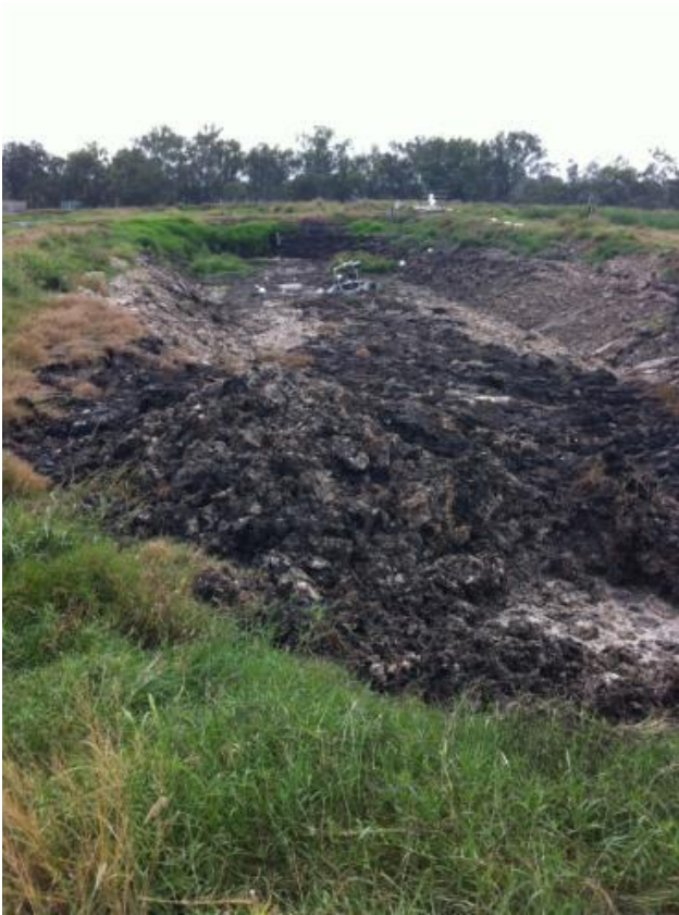
Figure 4.16: Pond A during sludge removal using a SludgeRat® sludge removal system. Removal of fat build up at the pond inlet (bottom of image).
