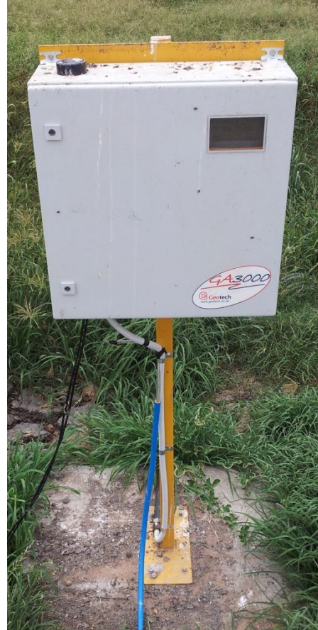
Figure 3.4: GA3000 gas analyser installation at northern end of pond B.
