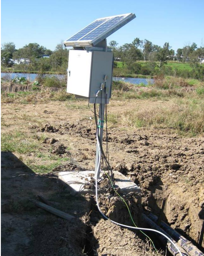
Figure 3.3: Instrument enclosure mounted at the head of Pond A
