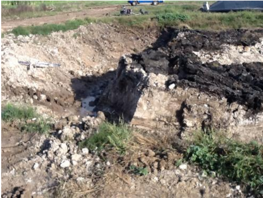
Figure 4.15: Section of crust removed by the excavator after sludge was pumped from pond A indicating crust thickness.
