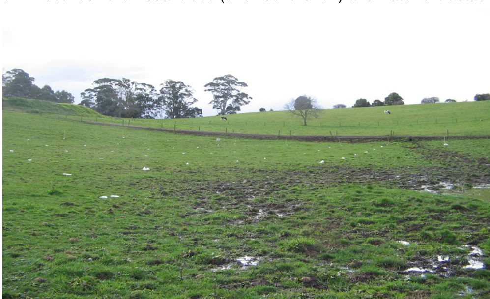
Figure 26: Site 2- Effluent leaking from effluent pond
