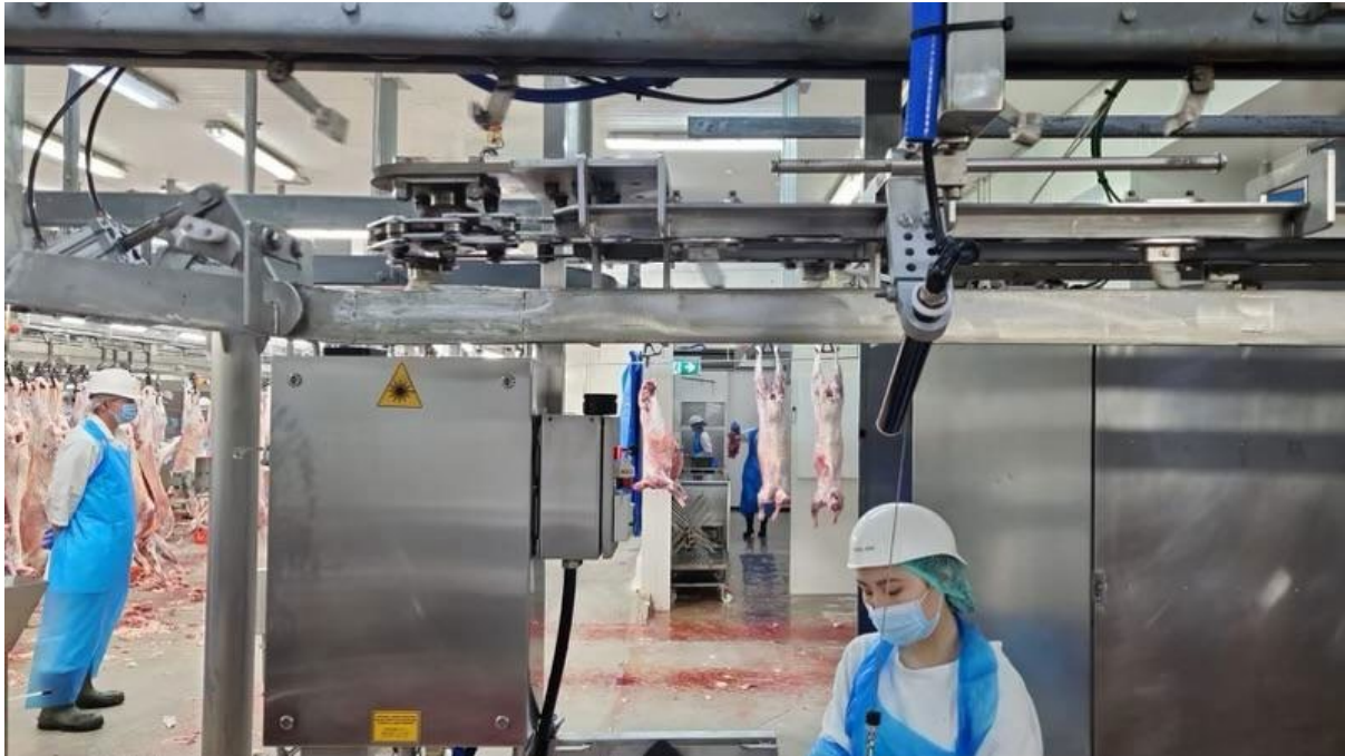
Photo 4. MEQ Probe fully installed at Frews with RFID reader in view.
