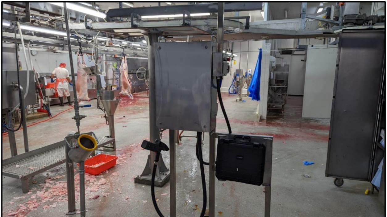
Photo 1. MEQ System installed in Frews Slaughter Floor
