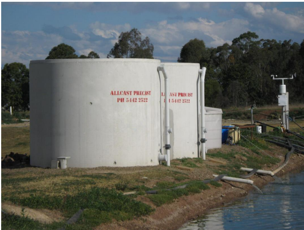
Figure 3: SAR Process installed on site in 2012
