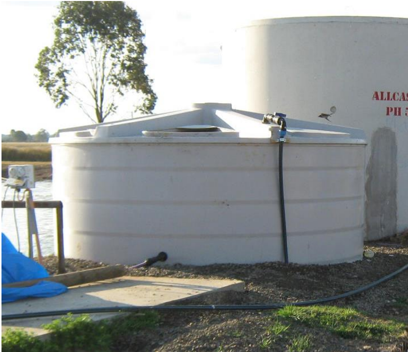
Figure 8: Filter Tanks with Regeneration tank in foreground
