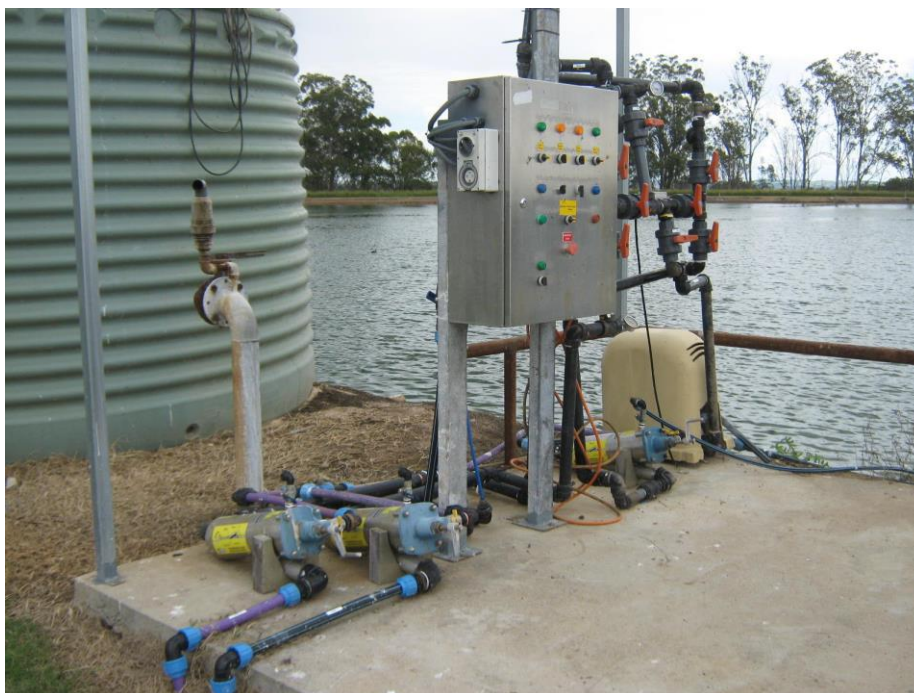
Figure 17: Pre-filter, Flow Control Valves and Power Control Systems installed November 2012
