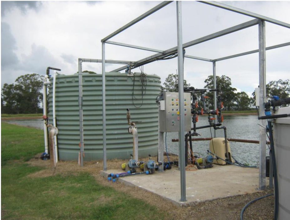
Figure 18: Settling Tank installed January 2013
