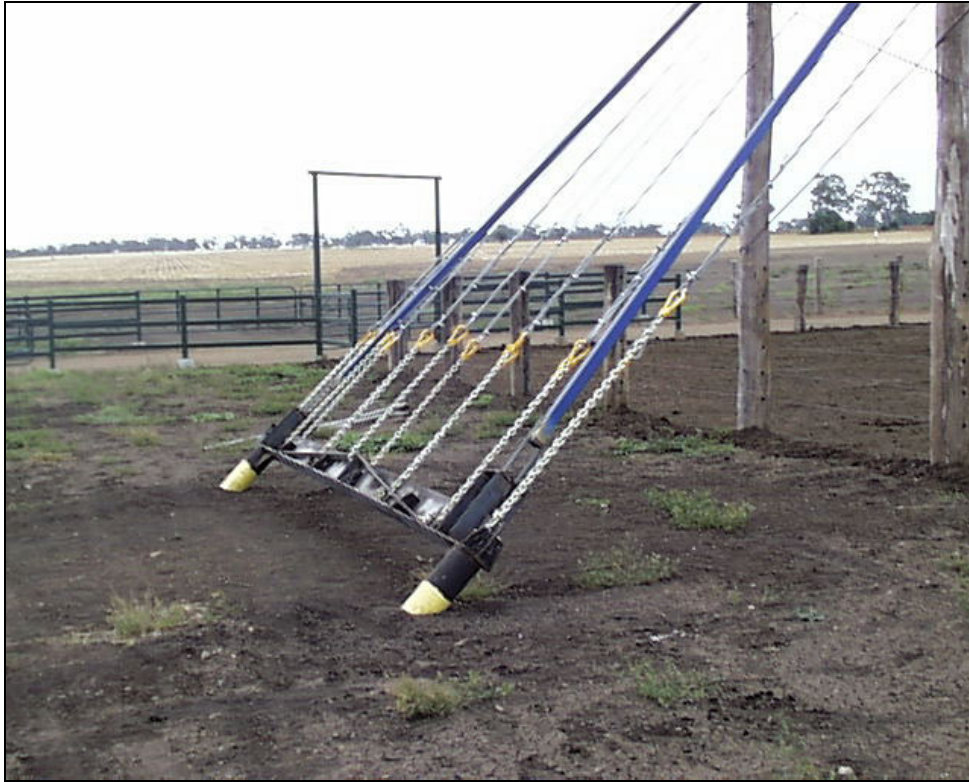
Figure 8. Anchorage and cable tensioning system seen for the shade structures at Feedlot B.
