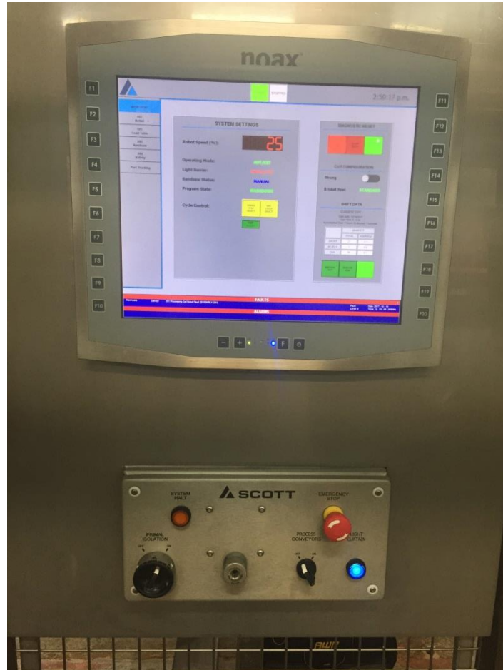
Fig. 5: Operator HMI and Controls
