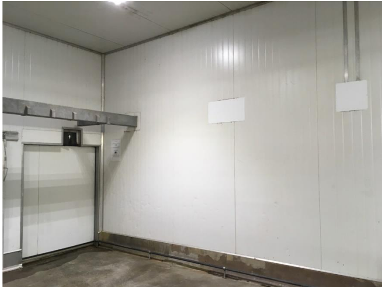
Fig. 1 Forequarter Machine Installation Room
