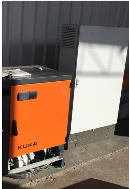
Fig. 8: Robot Controller and MCC
