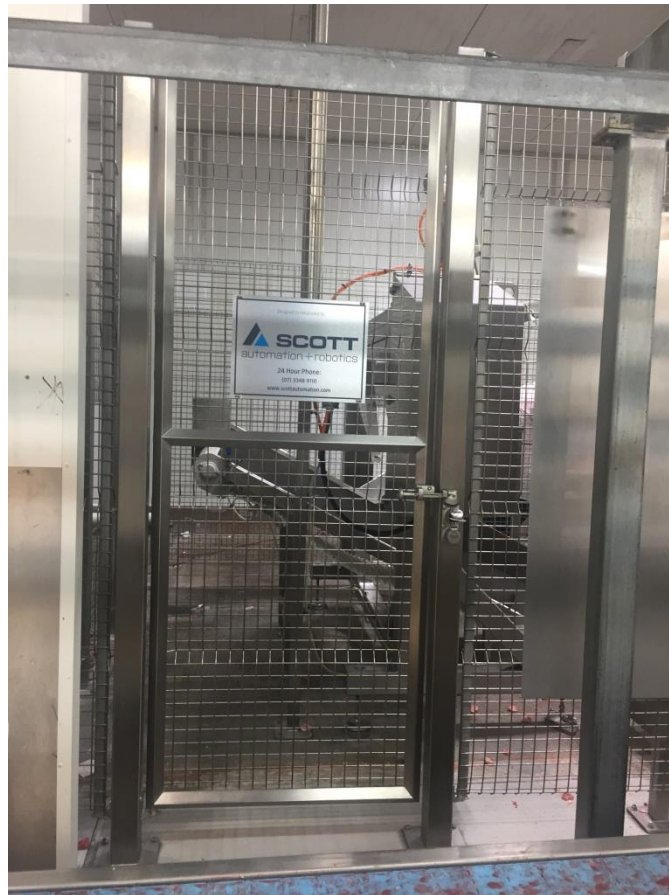
Fig. 7: Operator Access Gate
