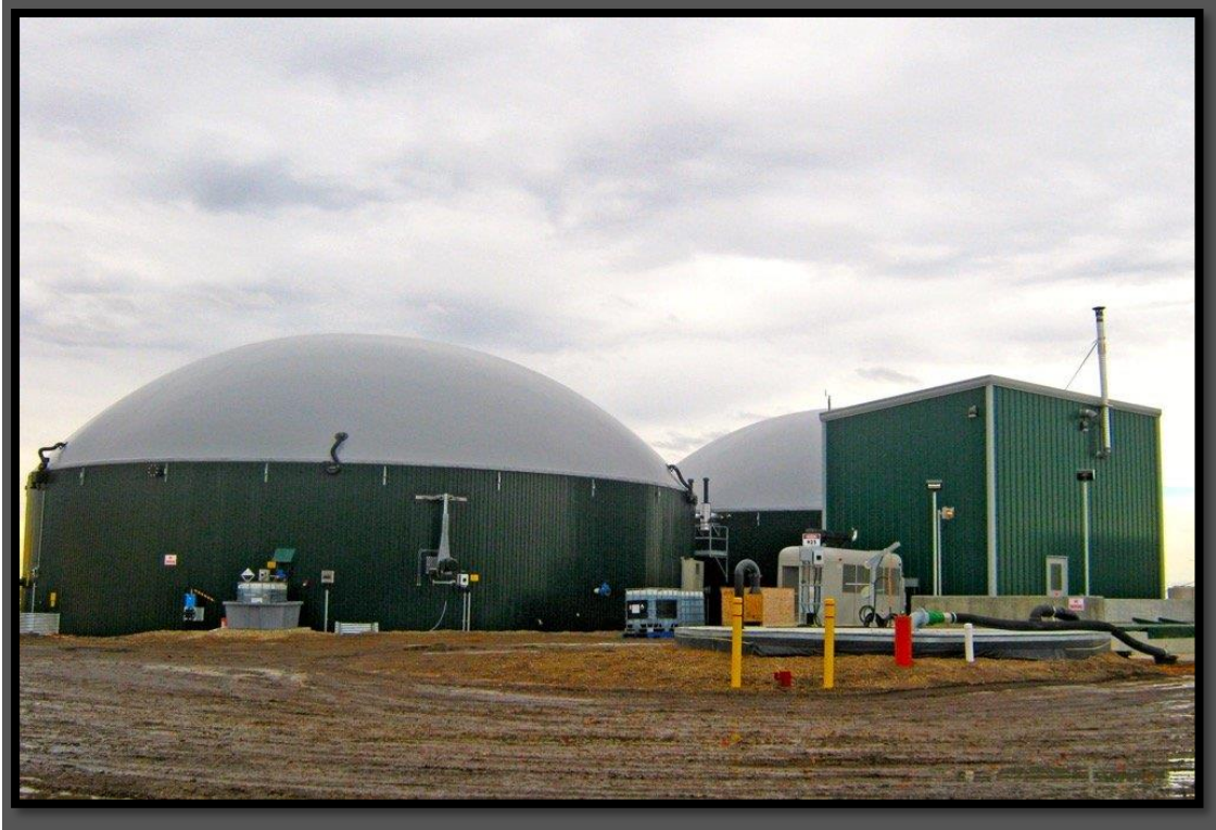
Figure 5: twin digesters at a Canadian feedlot produce 630 kilowatts of green power annually while reducing carbon dioxide emissions by more than 10,000 tonnes annually. The facility cost $CAD 7.1 million when installed in 2014 and can process 25,000 tpa of organics 28 .
