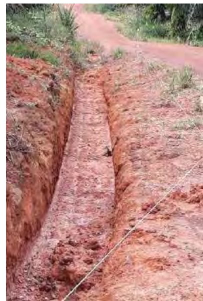
Drainage ditches and/or bunds on the upper side of the slope will divert overland flow away from the yard.
