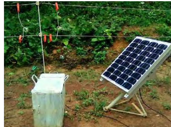
Electric fencing power box and solar panel
