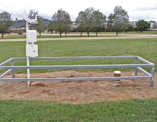
Well-sited 2 metre AWS with no nearby obstructions and a low security fence.
