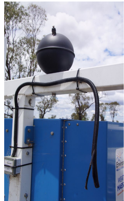
Well protected cabling on an AWS.
