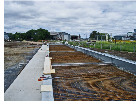
Weighbridge platform construction – concrete platform and reinforcing mesh needs to be well connected to the main lateral beams to prevent buckling.
