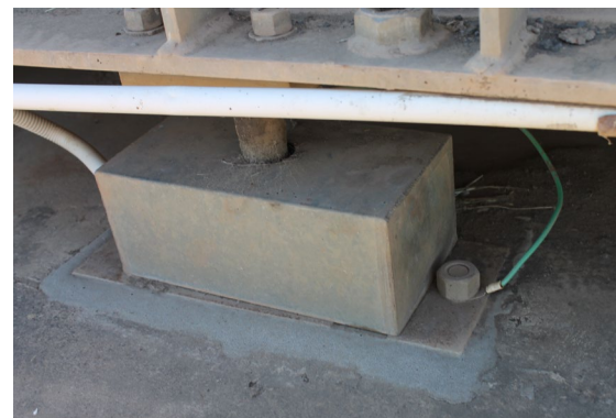
Load cell and weighbridge located above ground allows easy access for maintenance and re-calibration, and good drainage.
