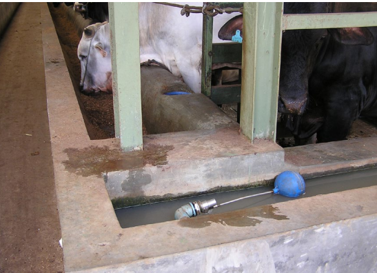
Unprotected floats can be damaged resulting in an overflowing trough and wet spots within the pens.
