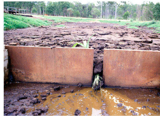
A vertical slot weir used in a sedimentation terrace
