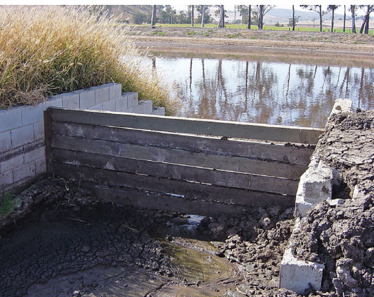
Sediment has built up between the walls of this control outlet as there is insufficient space for maintenance equipment to reach it. The control structure should have been located at the end of the block wall structure.
