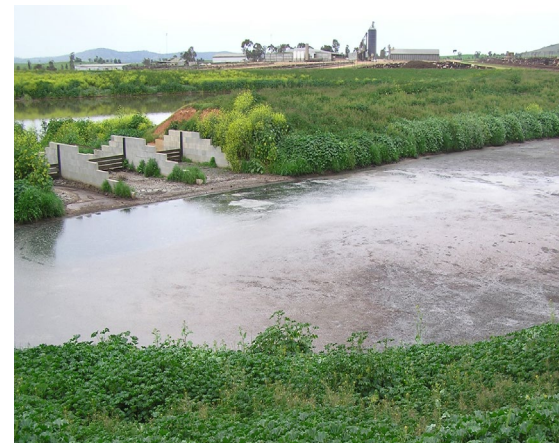
Upstream of the outlet control structure. Excessive removal of sediment has caused the floor of the basin to be lower than that of the control structure so the basin cannot fully drain. When removing sediment, do not alter the base of the sedimentation structure.
