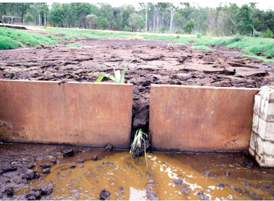
Solids have been effectively controlled. Now the system needs cleaning immediately.
