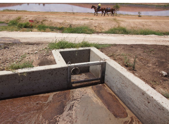
Where possible, solids and larger suspended matter should be removed from the effluent stream from hospital pens, cattle washing facilities and induction facilities with a coarse screen before the settling pond. The base of this area should be large enough to allow maintenance equipment to remove the settled sediments.
