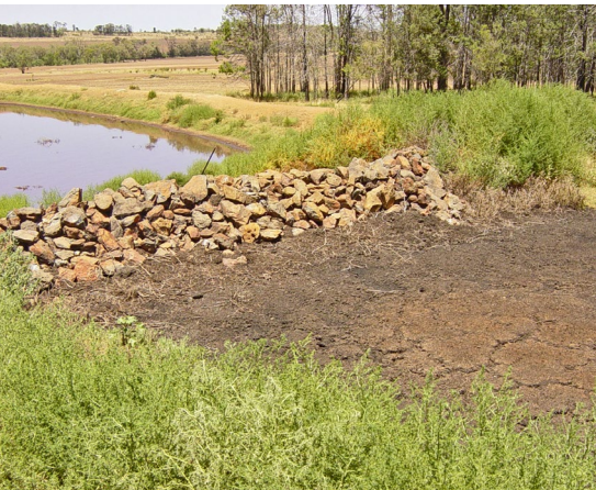
Rock-filled weirs are a poor design choice as they clog easily.
