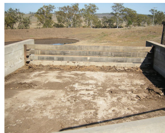
A typical horizontal timber drop-board weir. There should be a minimum freeboard of 900 mm between the control weir crest and the crest of the sedimentation system embankment.
