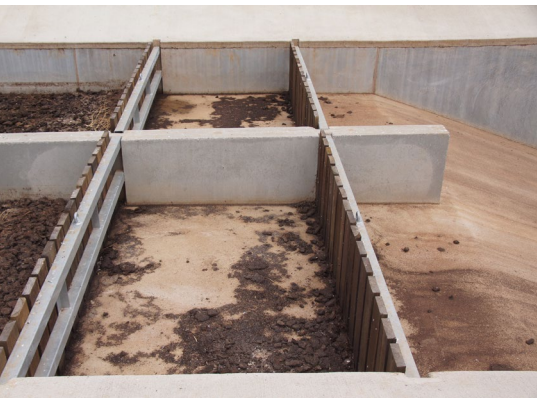
Typical vertical timber board weir, incorporating two rows of drop-boards and reinforced concrete base.
