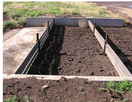
Horizontal timber slat control weir showing deposited sediment on the upstream side with little manure on the downstream side. The basin has drained completely and is drying out so that the solids can be removed.
