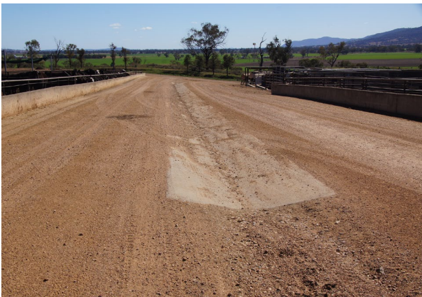
Drainage of feed roads showing slope towards the centre as in Option 1 of Figure 6.
