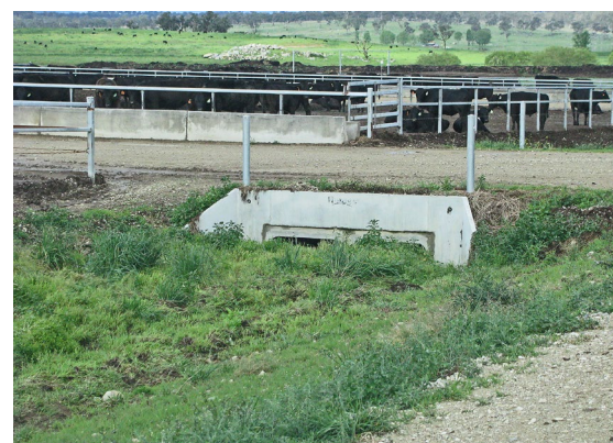
Sediment is deposited when vegetation reduces stormwater flow through culvert.
