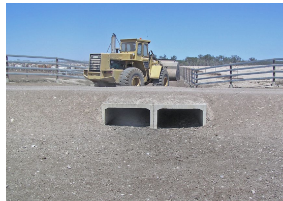
This concrete box culvert allows cleaning of settled manure in the drain on both sides of the culvert.
