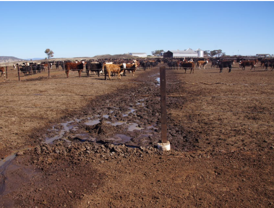
Pen to pen drainage is not desirable. Here a row of pens runs up the slope towards the feed mill with little cross slope. Runoff and manure flows through all pens before exiting at the lower end. This runoff is from a leaking water trough in a pen in the middle of the row.
