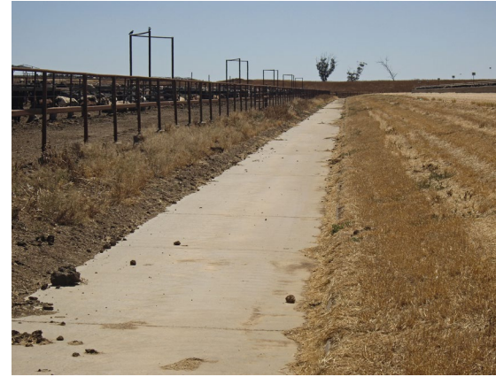
A well-maintained concrete drain within a feedlot. The dimensions of this drain allow access for cleaning equipment.
