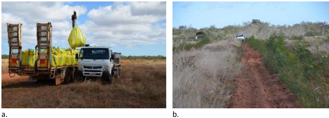
Fig. 9 Broadcast superphosphate application 1 August 2017; a. approx. 15 t of fertiliser delivered to site, b. application in progress (Paddock 4 – Redlands).
