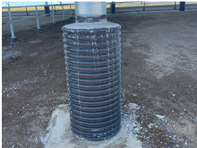
Photograph 23: Ribbed HDPE poly pipe protective hob
