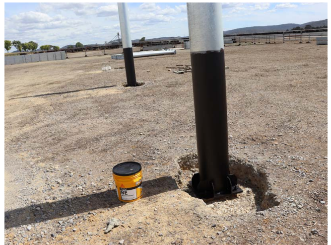
Photograph 22: Building support column with painted bitumen emulsion treatment
