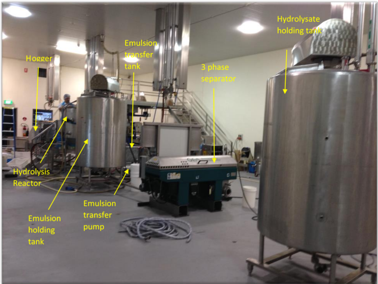
Figure 3 Hydrolysis trial equipment layout
