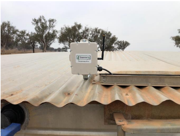
Figure 5: Redbank water tank sensor
