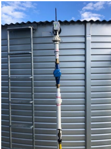
Figure 10: Redbank water flow sensor
