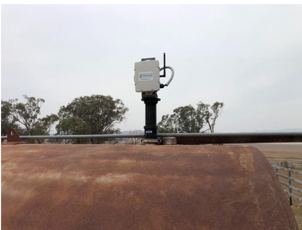
Figure 6: Redbank diesel fuel tank sensor
